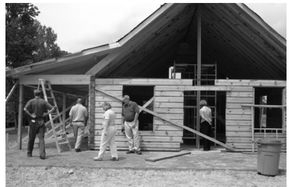
Ronald Bennett guides a tour group through the construction of a new retreat facility on his farm in Vance County.
