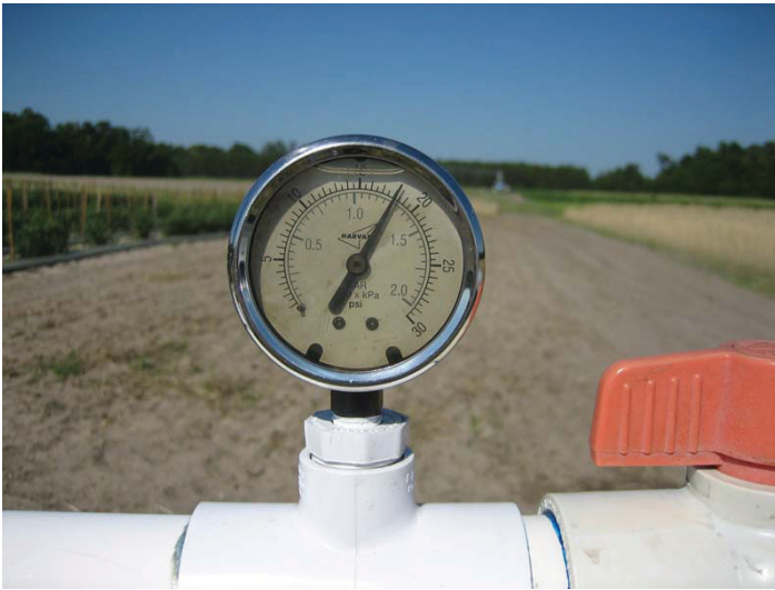
Figure 10. A fixed pressure gauge. Note the needle bathing in oil to prevent needle vibration and damage. Credits: Eric Simonne.
