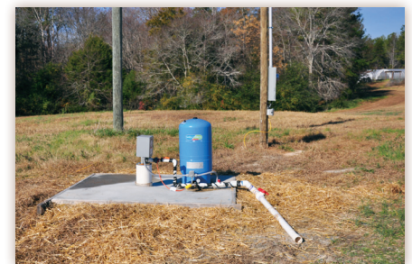
▲ This well has a concrete pad to help minimize the risk of contamination.
