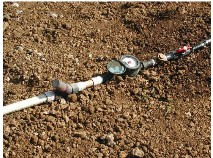
Figure 8. Water meters installed near the field.
