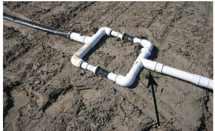
Figure 7. Pressure regulators are installed side-by-side in this system to allow a greater flow rate. Note the small injection port for chemical injection.
