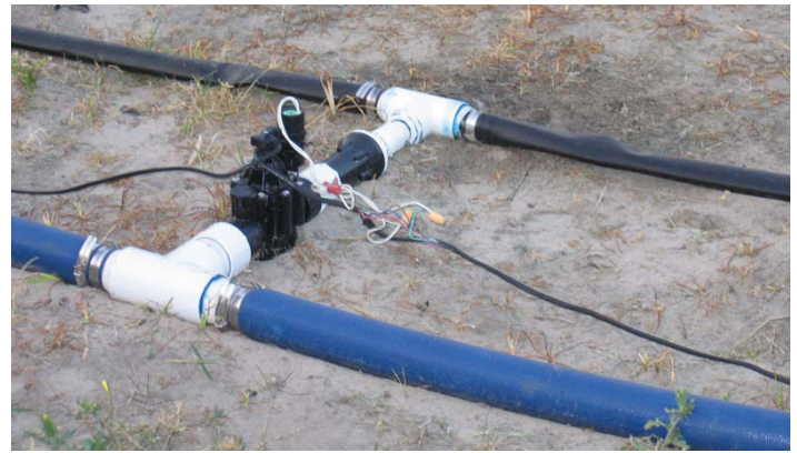
Figure 11. Solenoid valves connected to a timer allow sequential irrigation of different zones. Credits: Eric Simonne.
